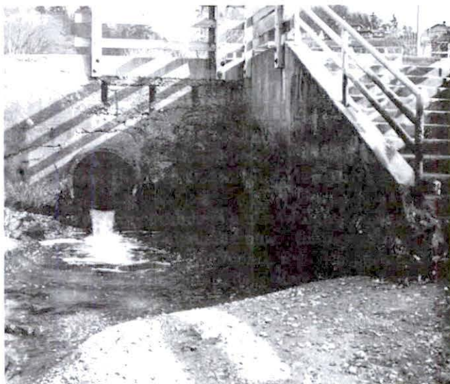
Redondo Creek empties into Puget Sound via a culvert south of Salty's Restaurant.
